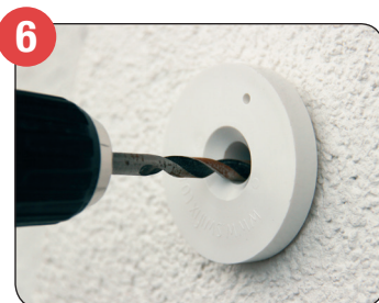
6 Drill through tube into substrate to the appropriate depth for fixing (you may require the use of the washer supplied, dependant on fixing used).
